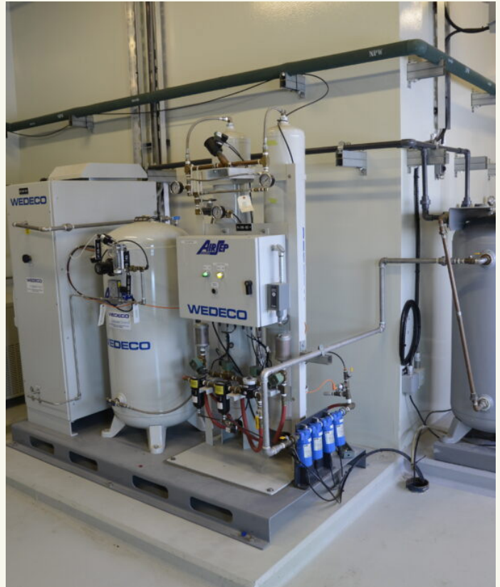
Xylem's ozone oxidation equipment, used to produce Alberta's first beer made with reused water, created an effective barrier for removing viruses and bacteria from the water stream to disinfect it. Photo: Xylem Inc. (from Water Canada ).
